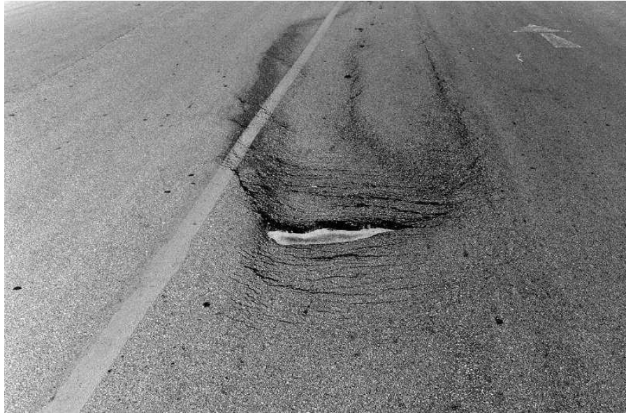
Figure 1.1. Slippage cracking (Asphalt Institute, n.d.).
