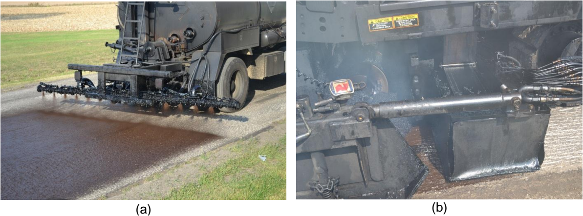
Figure 3.11. (a) Tack coat application with distributor truck, (b) Tack coat application with spray paver.
