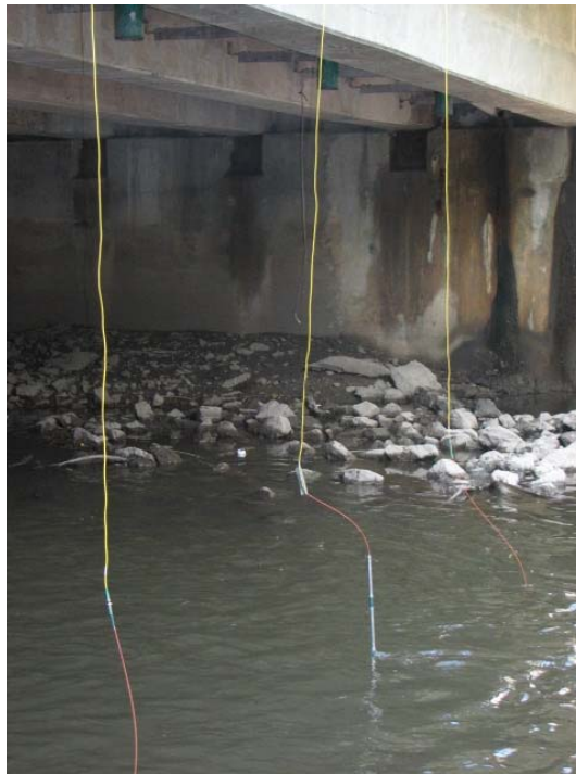
Figure 12. Three sensors installed on June 23, 2008.
