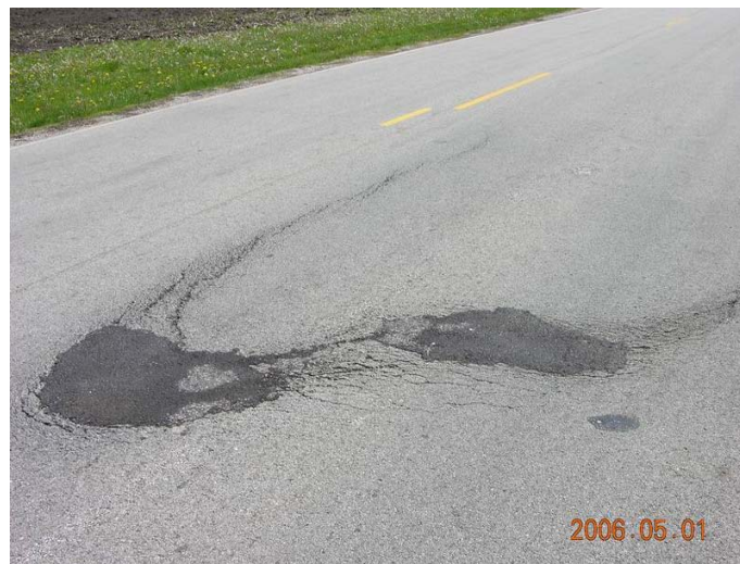
Figure 1-1. Slippage cracking caused by poor interface bonding.
