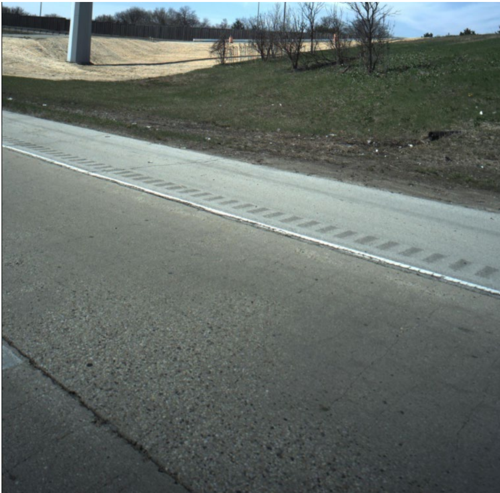
Figure 10. Image. IROADS image of transverse cracks in right driving lane with light pole, pavement stripes, shoulder grooves, and pavement width as reference distances.
