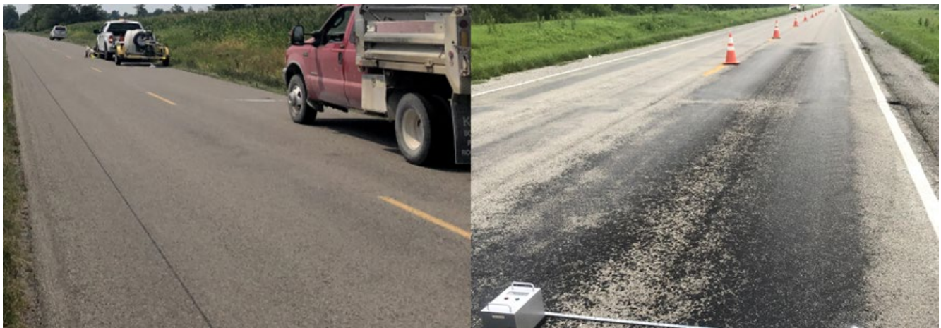
Figure 5. Photo. Chip seal surfaces from the test sites showing a newly constructed site in good condition (left) and one site with excessive bleeding (right).
